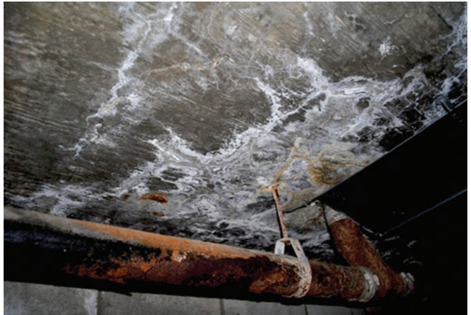
Water intrusion through the concrete garage ceiling, resulting in damage to plumbing lines and attachments.
