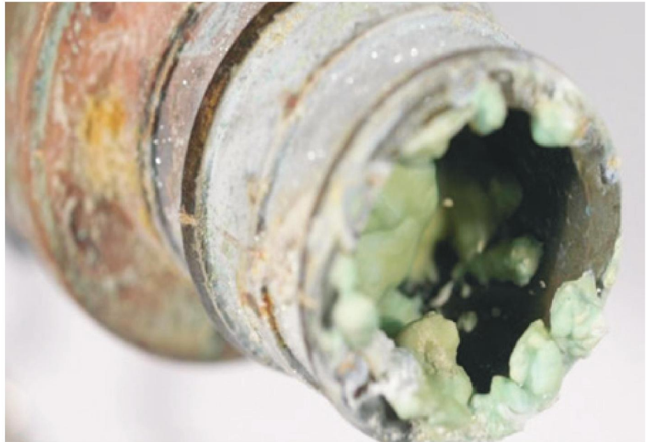
A PEX, yellow brass fitting, attaching the PEX tubing to a copper water line. The fitting is badly dezincified, with a substantial meringue deposit inside the fitting, as well as on the barbs which lie between the fitting and PEX tub.
