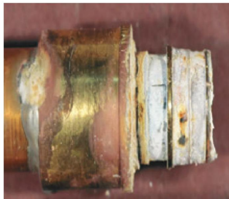
A PEX fitting with the copper water line removed showing corrosion on the barbs and significant deterioration of the fitting itself.
