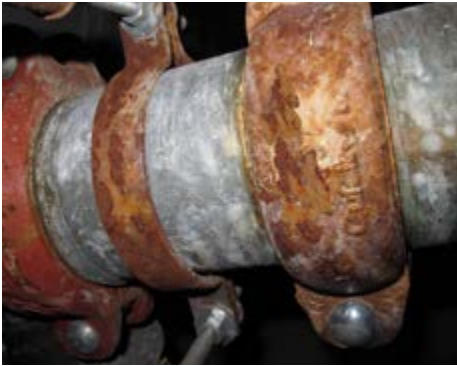
Waterway fitting corrosion
