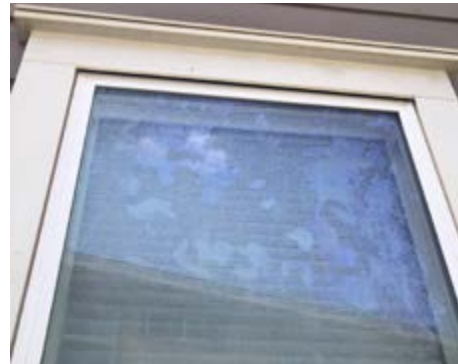
Low E coating failure
