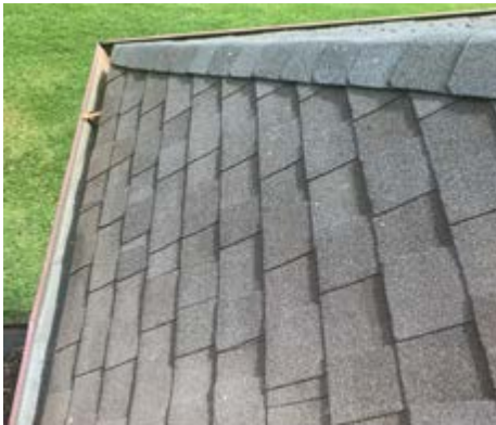
Asphalt shingle deformation
