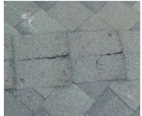
Asphalt shingle cracking
