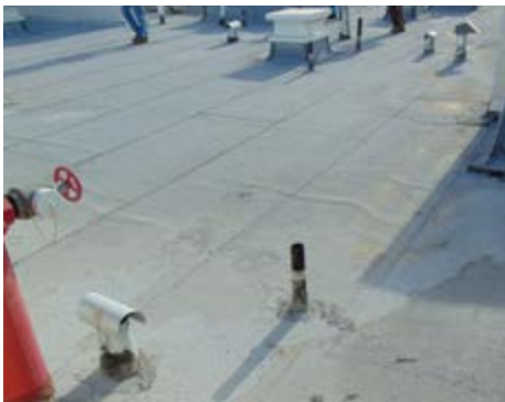
Built Up Roof bubbling and deterioration
