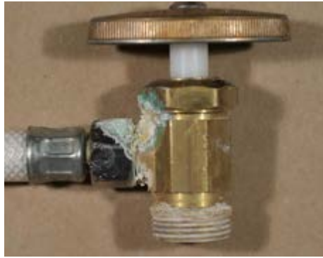
Angle stop corrosion
