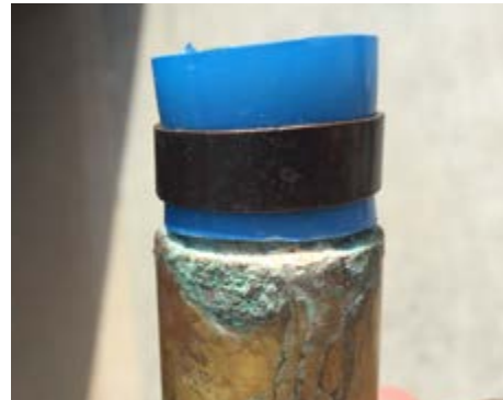
PEX fitting corrosion
